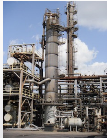
Sour Water Stripping Unit
