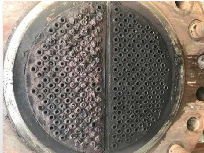
BFW / HT heat exchanger bundle before chemical cleaning process
